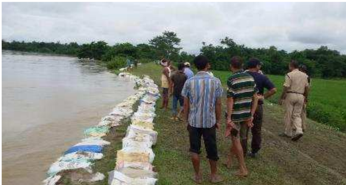
Overtopping of Dyke of Buridehing river
