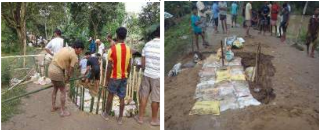
Damages due to sudden slump down of dyke structure die to seepage, leakage etc.
