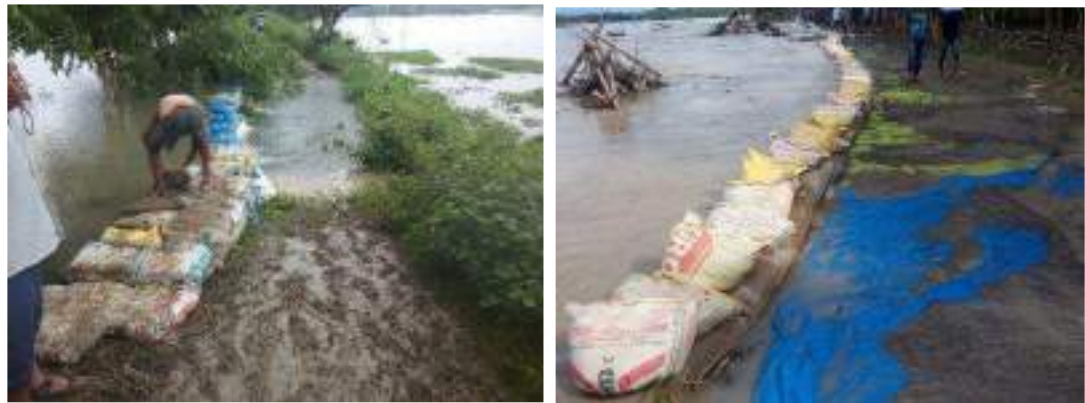
Overtopping of the dyke
