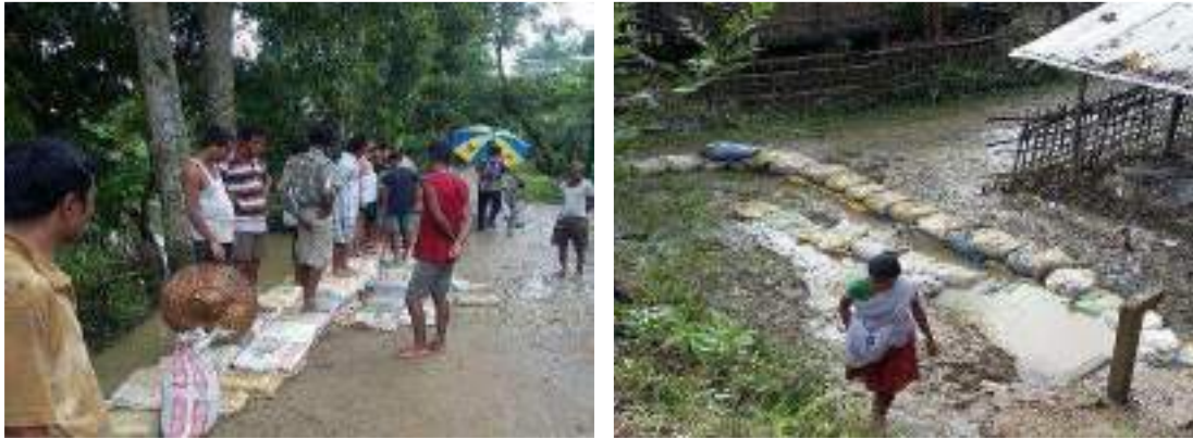
Overtopping and seepage, boiling leakage etc.
