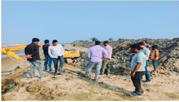
Site Visit at to take note of the work progress Baramari Gaon, Morigaon
